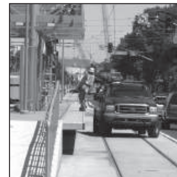
Workers put the finishing touches on the Third Street light rail extension.
